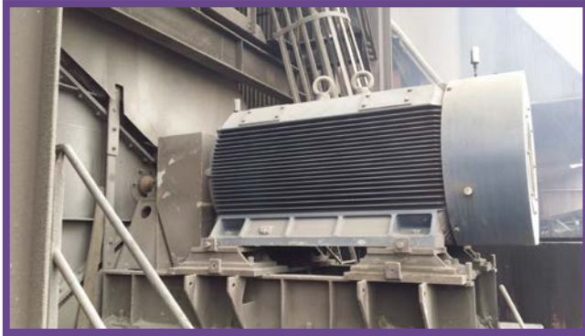
The two high voltage Marathon electric motors each weighing over five tonnes and rated at 900 kW have been installed to replace two fan motors in the exhaust gas stack that failed at a prominent metalliferous process plant in Tasmania.
